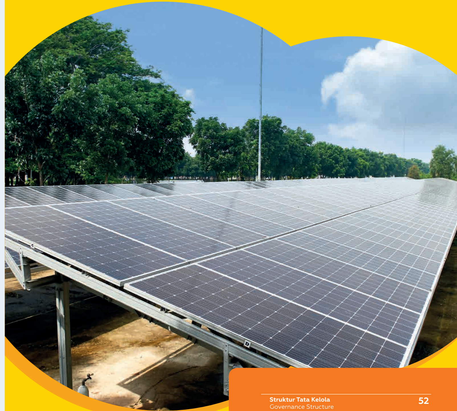
Teknologi Solar Photovoltaic di Kawasan Pabrik Karawang 1 Photovoltaic Solar Technology applied at Karawang 1 Manufacturing Plant area
